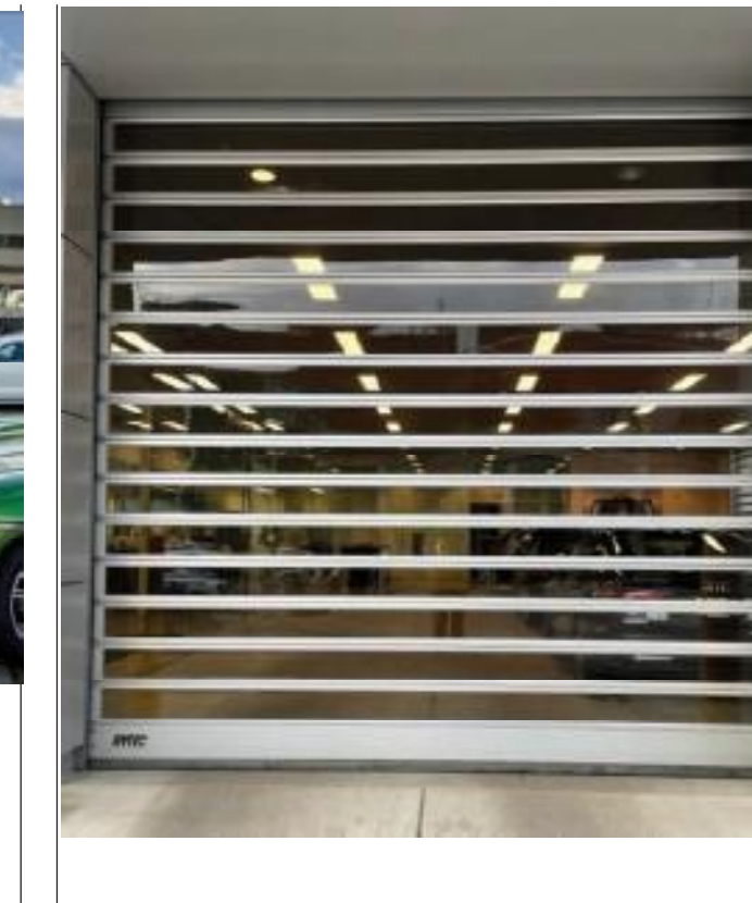
K OVERHEAD DOORS
