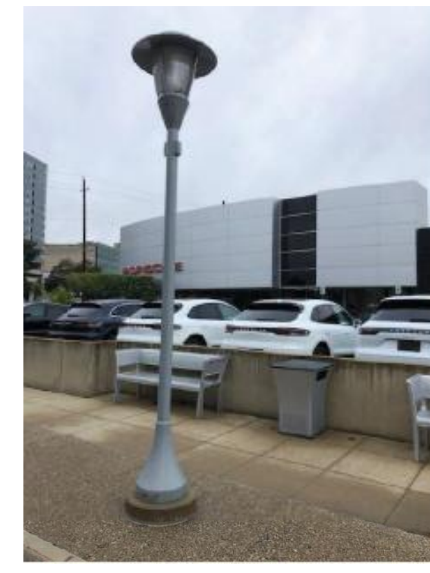
E EXISTING & NEW STREETLIGHTS (S-47 & S-24) Luminaire Street Light Model P190-42-V To conform with Triangle District Standards
