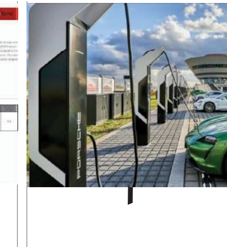
J CHARGING STATION (AC) 2 Public Accessible located on Haynes Street
