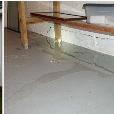
There are large cracks in the foundation and extensive leaking in the basement.
