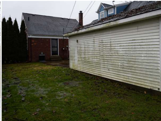
The garage is covered with mold.
