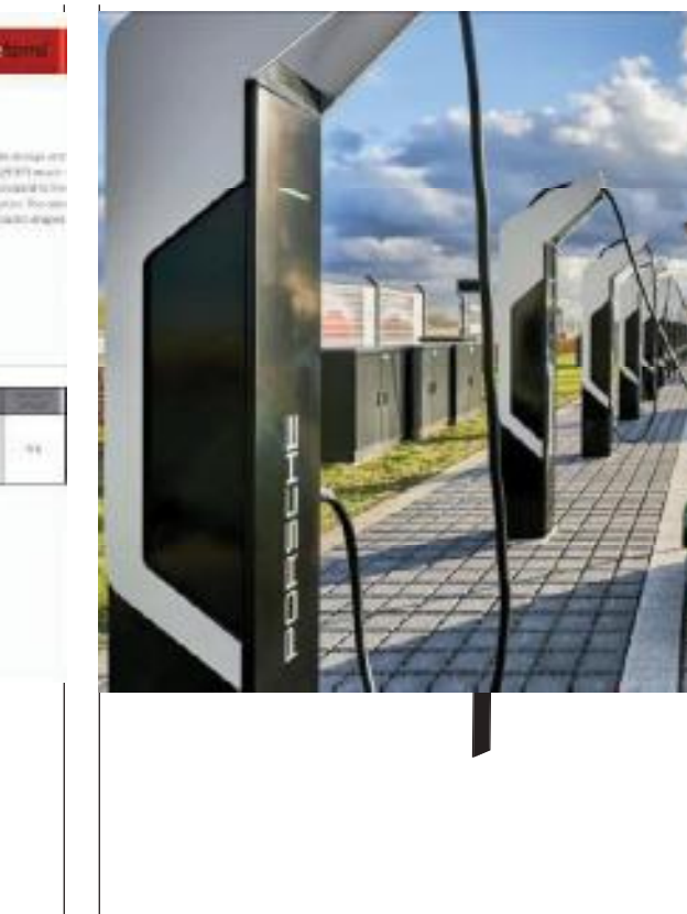
J CHARGING STATION (AC) 2 Public Accessible located on Haynes Street
