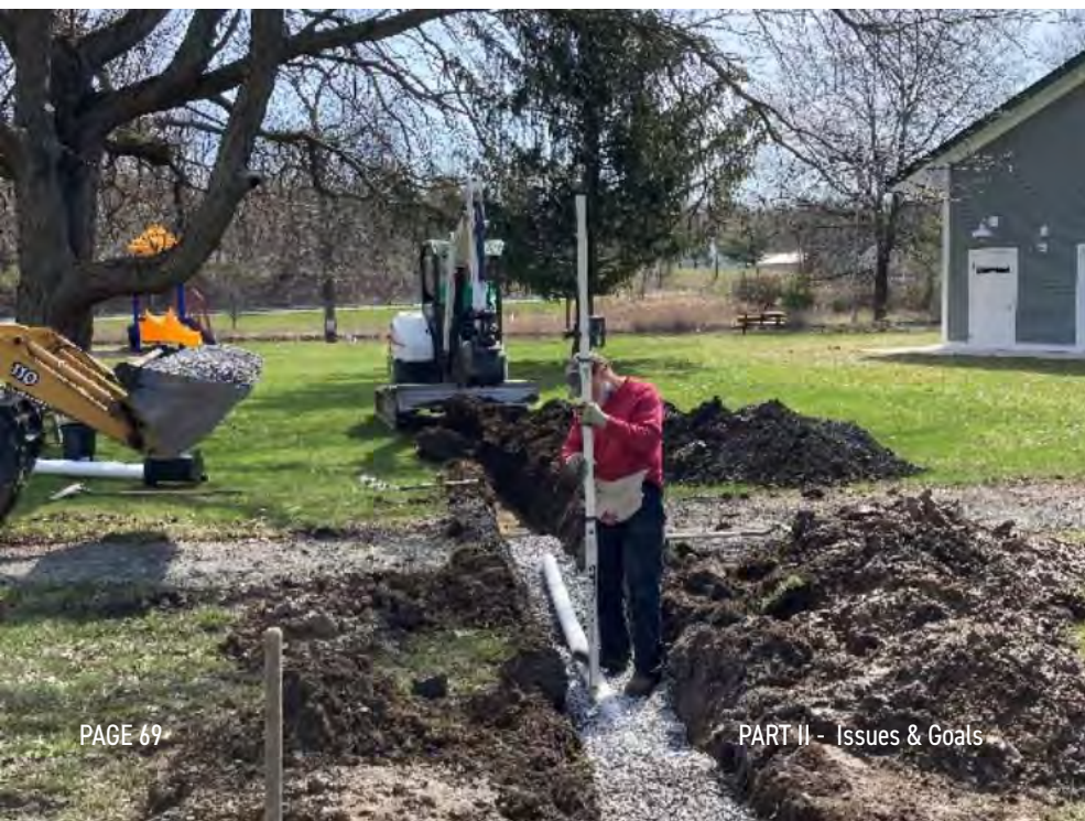
Maintenance Work. Jim Klinger works to install new drainage pipes at Crellin Park to help address recent stormwater drainage issues.
