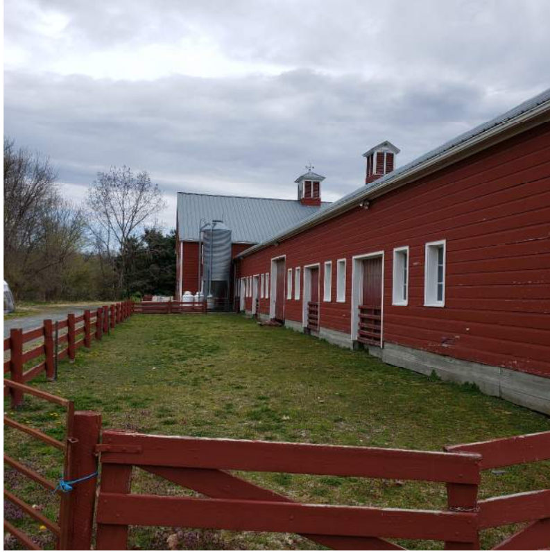
PHOTO 5: REAR (NORTH SIDE) OF BARN 1 EXTERIOR LIGHTING
