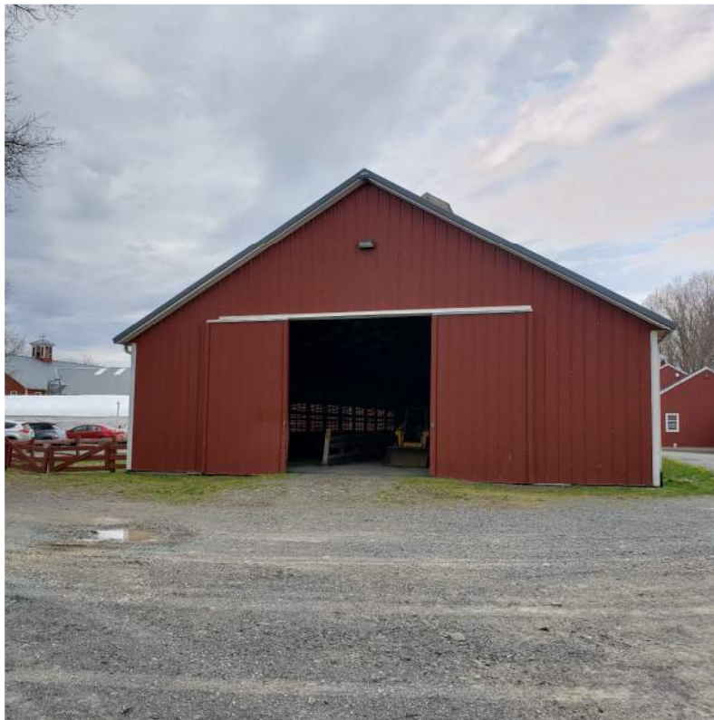
PHOTO 16: REAR (NORTH SIDE) OF BARN 4 EXTERIOR LIGHTING
