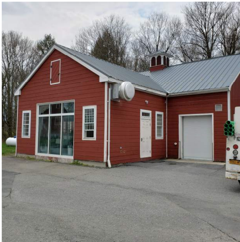
PHOTO 10: NORTH SIDE OF BARN 3 EXTERIOR LIGHTING
