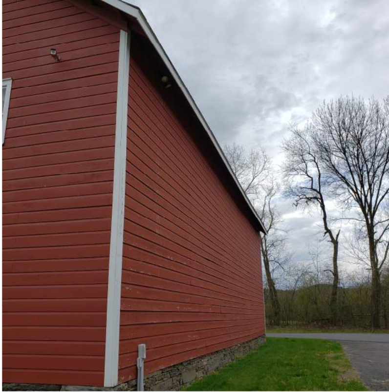
PHOTO 9: WEST SIDE OF BARN 2 EXTERIOR LIGHTING
