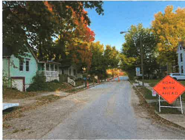
Commonwealth Ave. at Cambridge Ave. looking northwest. The intersection is the last remaining portion. Aprons are prepped for concrete.
