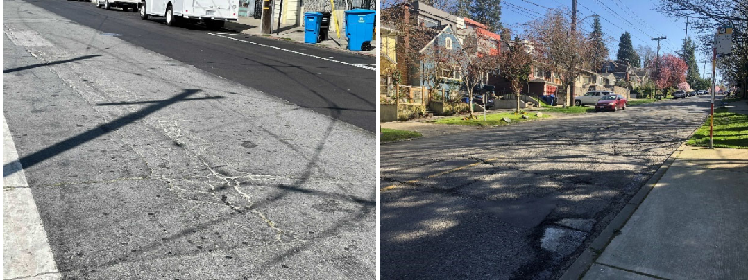
Figure 4-8 Asphalt Damage from Long-Term Heavy-Duty Transit Bus Use
