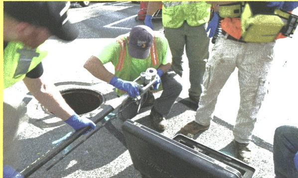
Sewer Operations technicians prepare a closed circuit TV camera to look for prohibited discharges such as fats, oils and grease.
