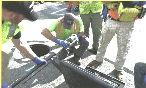
Sewer Operations technicians prepare a closed circuit TV camera to look for prohibited discharges such as fats, oils and grease.
