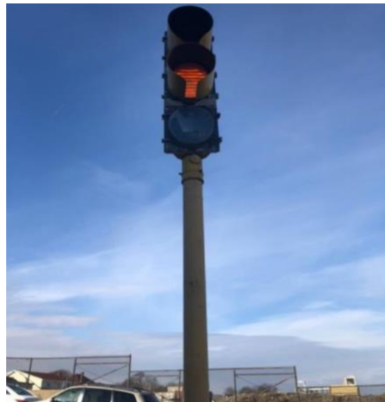
Figure 12 - Flashing yellow facing the wrong direction (Old Colony Avenue)
