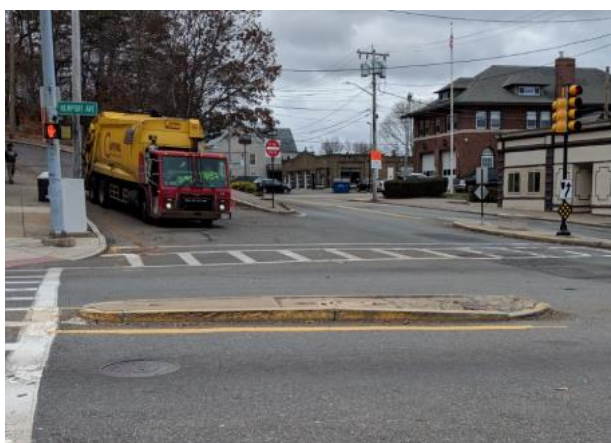
Figure 8 - Damaged median island on southern leg of Newport Avenue
