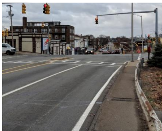
Figure 17 - Narrow sidewalk with guard rail on east side of Newport Avenue northbound approach.
