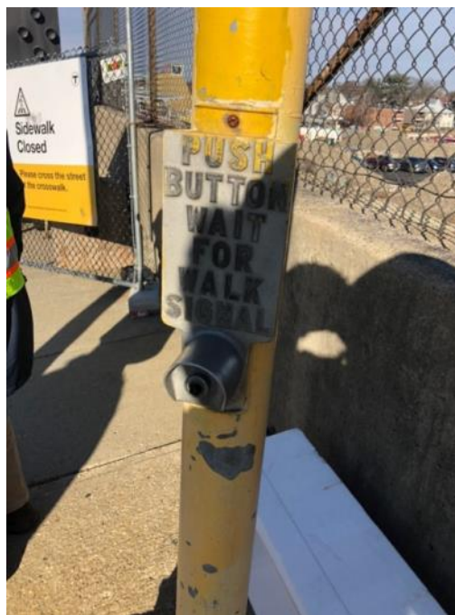
Figure 16 - Non ADA Compliant Push Button
