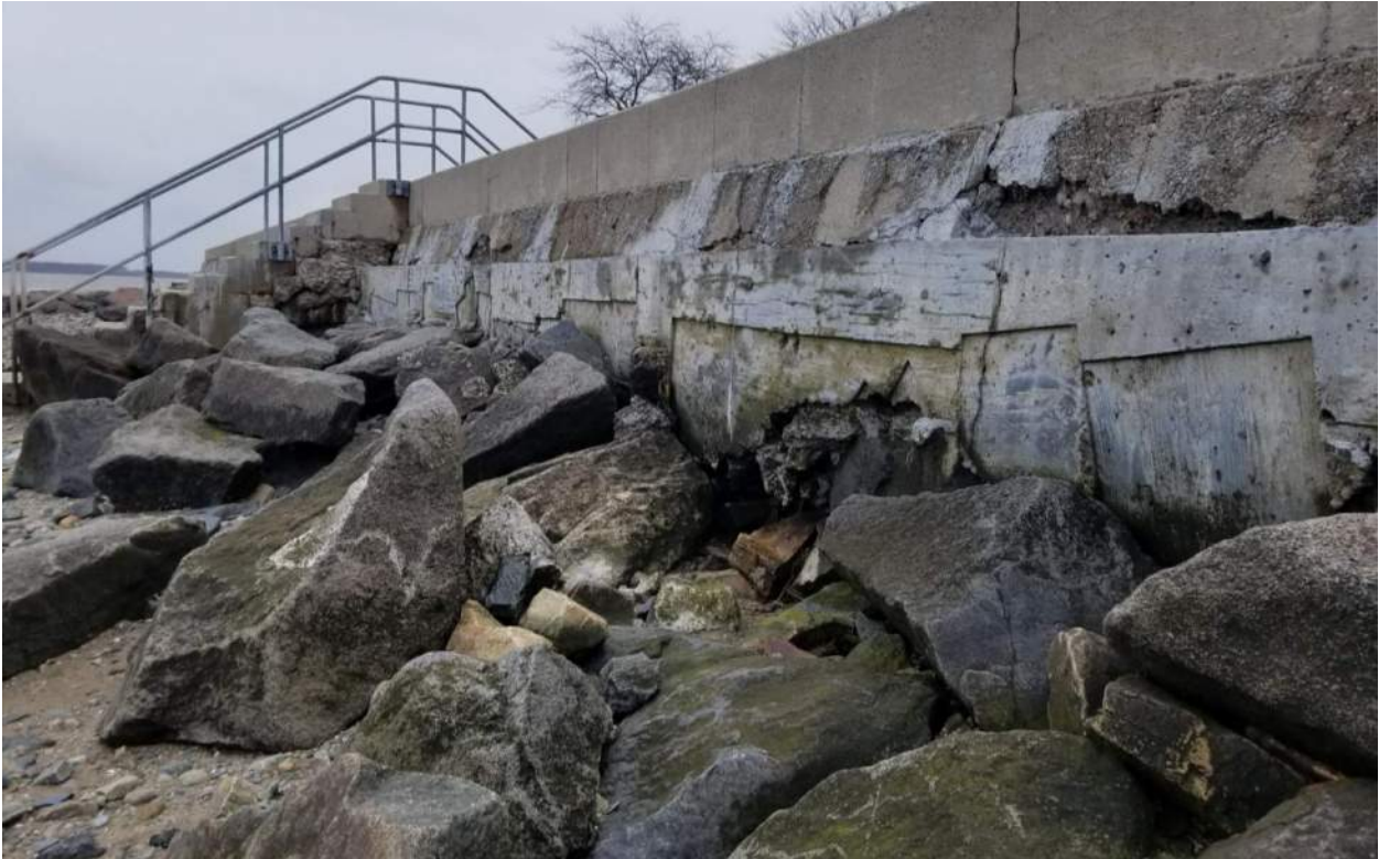
Photo 24: Dislodged revetment near the intersection of Crane Road and Shellton/Terne Roads, post-Winter Storm Riley (3/4/18).
