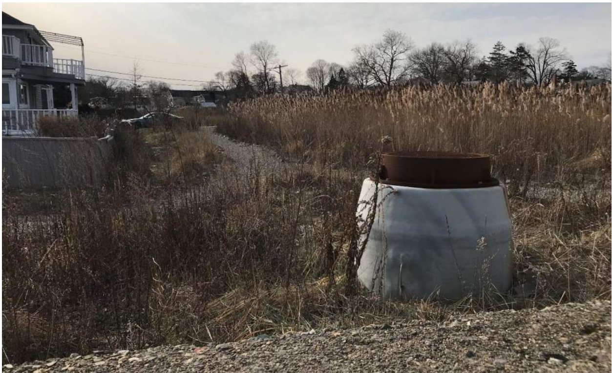
Photo 13: Looking south at a manhole structure near the salt marsh west of 5 Post Island Road (12/14/17).
