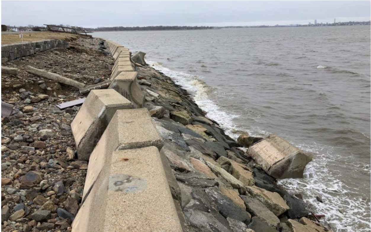
Photo 22: View looking west-southwest at dislodged seawall units off Shellton Road, post-Winter Storm Riley (3/4/18).
