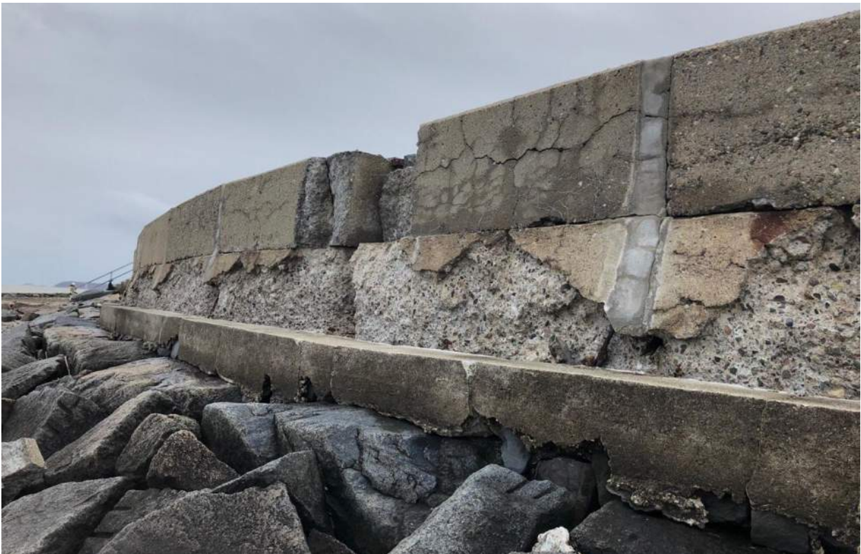
Photo 25: Seawall spalling off Terne Road, post-Winter Storm Riley (3/4/18).
