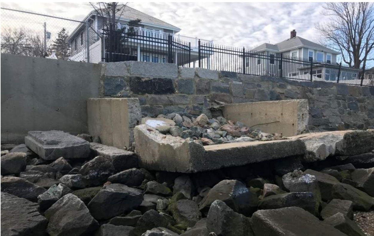
Photo 32: Photo of broken concrete wall (private), looking west-southwest near 48 Norton Road (12/14/17).
