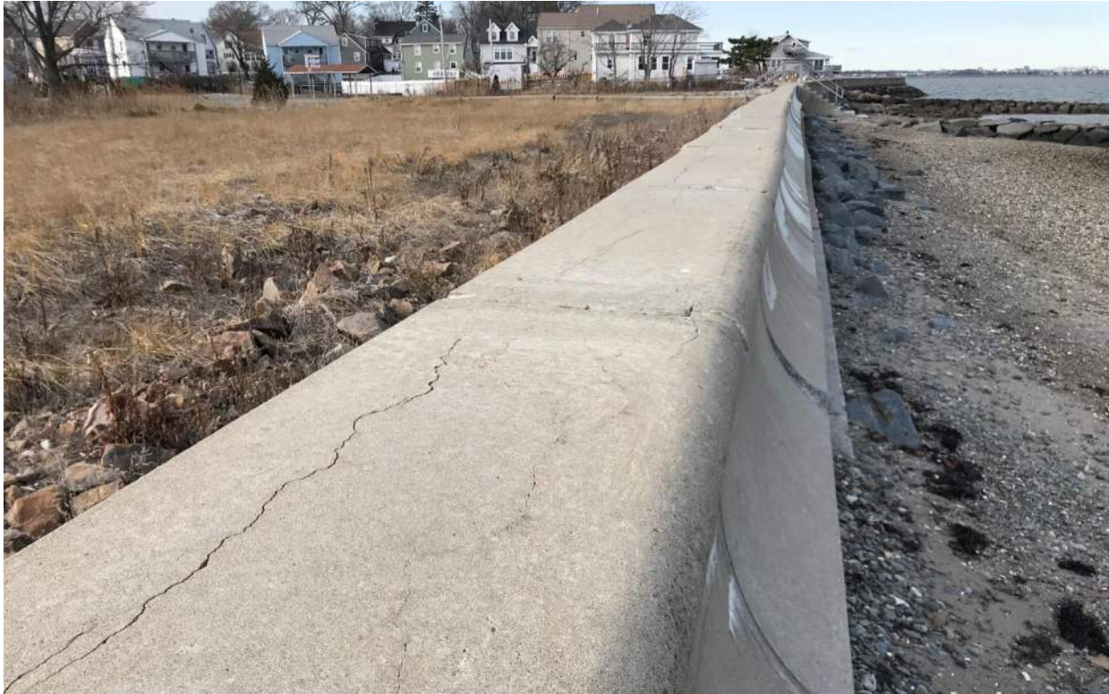
Photo 14: View looking northwest at the seawall, revetment, and rip-rap behind the wall; Arthur Boyson Park is in the top of the photo (12/14/17).
