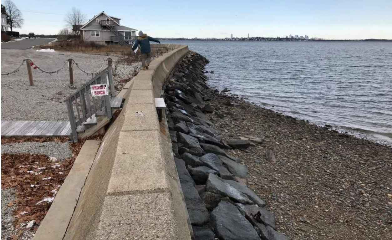
Photo 16: View looking northwest at seawall, revetment, and stairs near Mallard Road (12/14/17).
