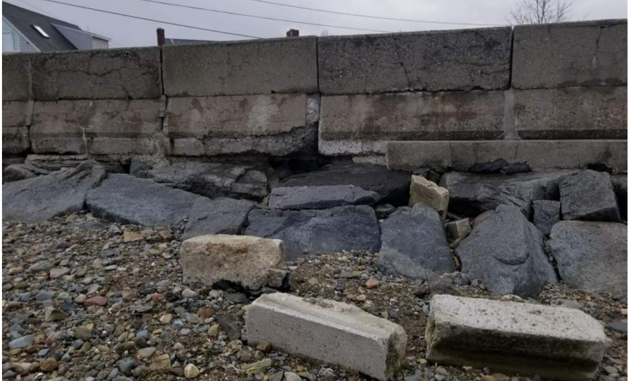
Photo 25: Leveling pad failure off Terne Road, post-Winter Storm Riley (3/4/18).
