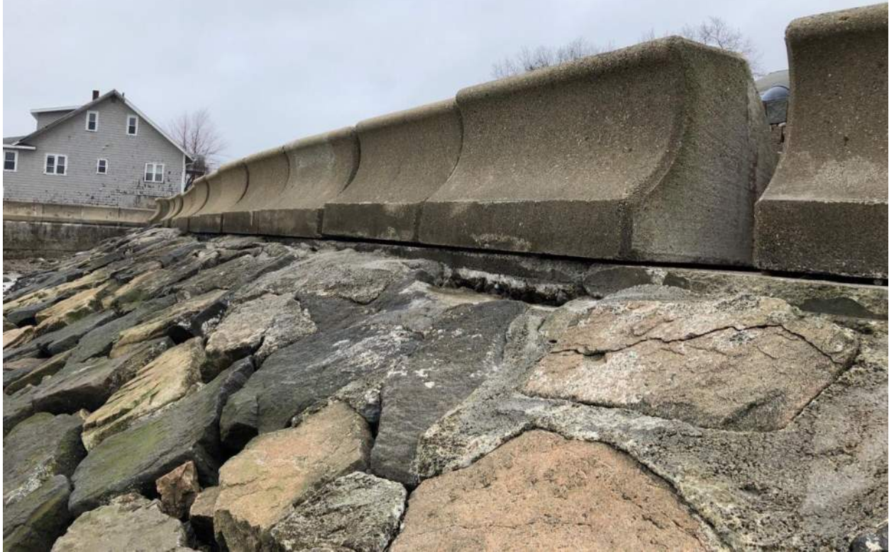
Photo 18: View looking southeast toward 72 Shelton Road at shifted seawall units and dislodged revetment, post Winter Storm Riley (3/4/18).
