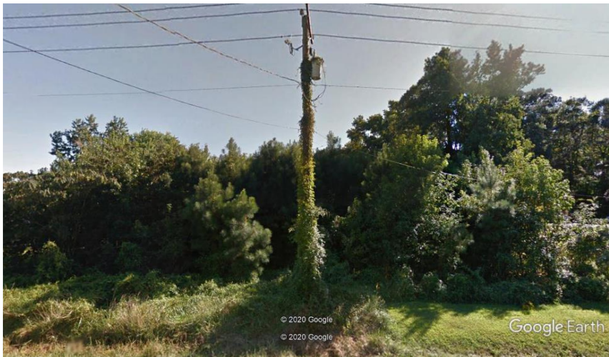
Figure 15: Utility Pole Requiring Make-Ready
