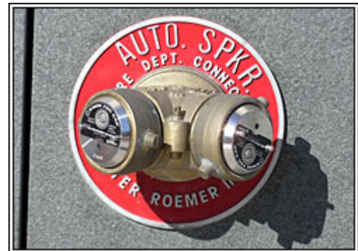
Example of a properly protected FDC
