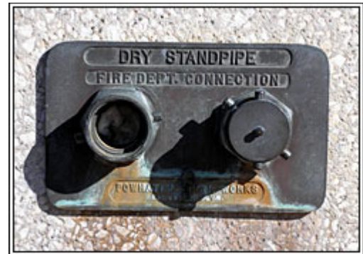
Example of a vandalized FDC with a missing cap
