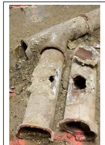
Broken sewer line Source: Unknown
