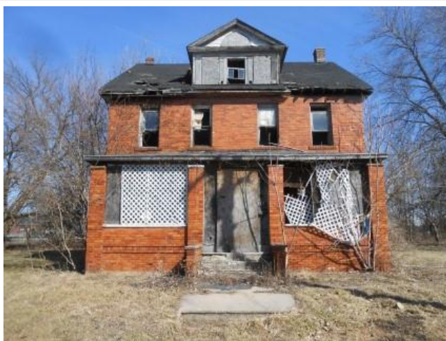
Property in Canton that was demolished through the Land Bank Source: SCLRC
