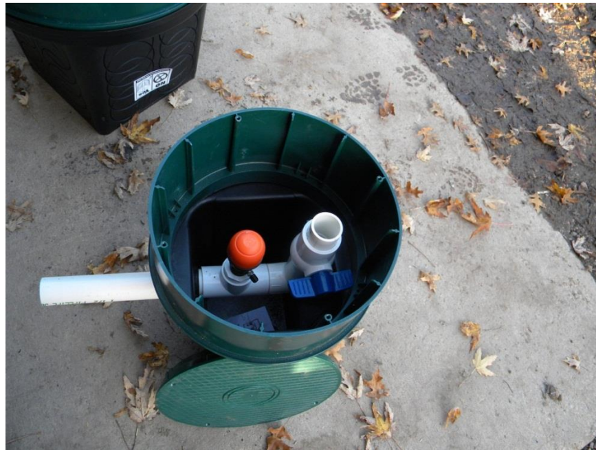
Figure 8. Turn-up and 3/4 inch air gap/ bleeder at the end of each lateral for routine maintenance
