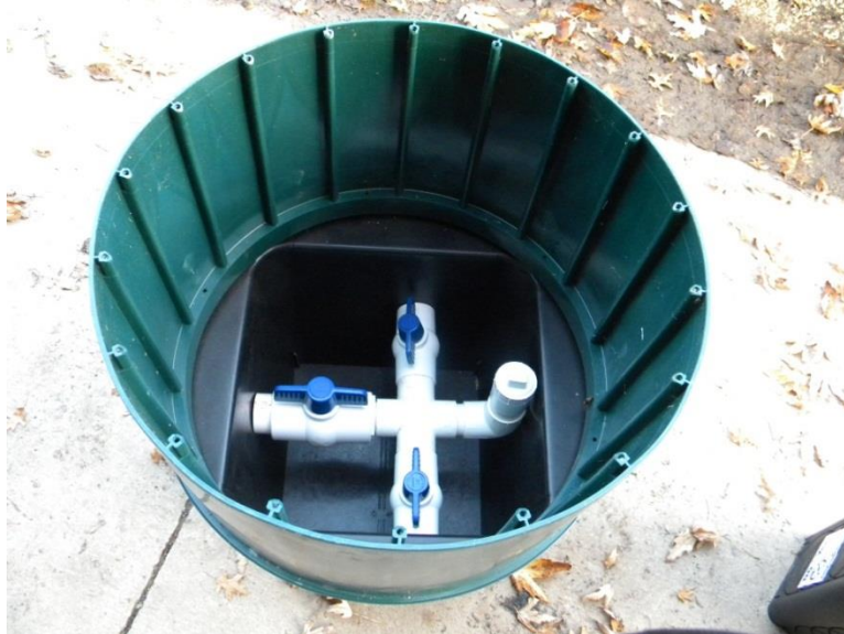
Figure 7. Service box within the manifold line
