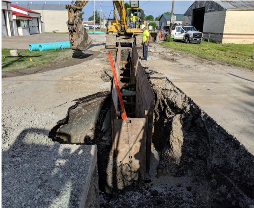
8-inch sewer main in roadway
